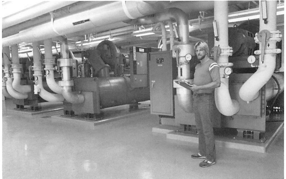
3,360 TON CHILLERS cool the water used in conditioning the air. Steve Williams, pictured here, is a senior engineering aide working for Operations. He has the responsibility for this new system.
